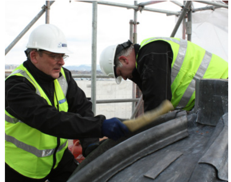
Author, Mike Maskrey (left), working on the lead-covered cupola of Stockport Workhouse
